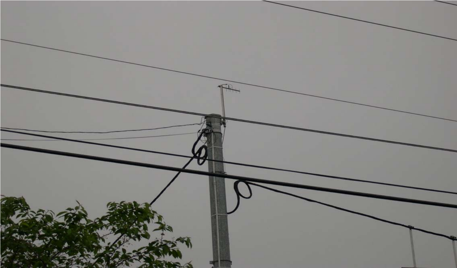
Radio Antenna at the Intersection of State Route 228/Heritage Creek Boulevard
